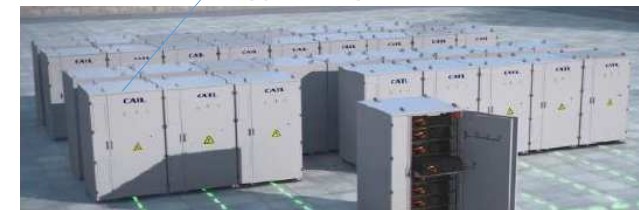
Energy storage (ENERDIGIT)
